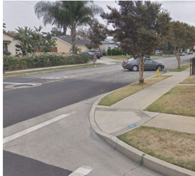
Visually non-compliant curb ramp, street view
