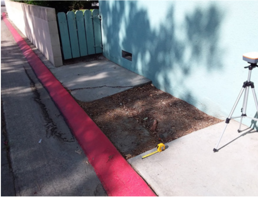
FIGURE 2-10: Missing sidewalk panel
